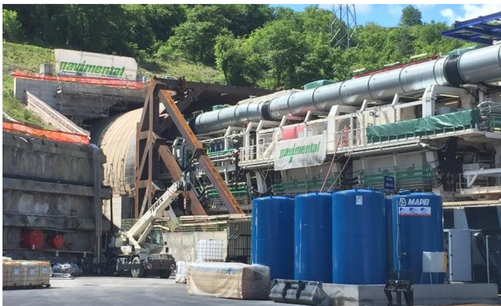
Image 4. Polyfoamer ECO/100 is delivered in bulk and stored on site in MAPEI tanks.
